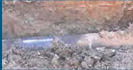
The full condition of the pipeline is verified once it is excavated
