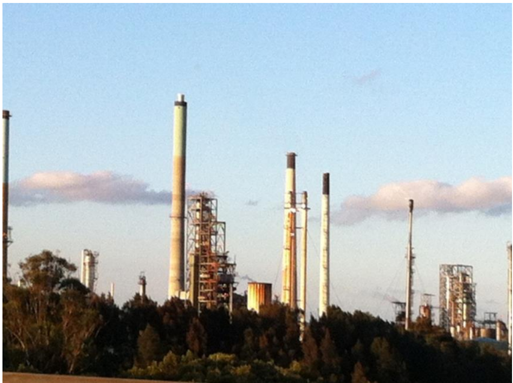
Plate 17 Views of the Clyde Terminal from the M4 Western Motorway toward the Project Area
